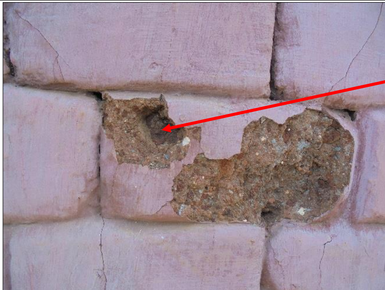
Poorly made ISSB's without sieving the soil eroding later.
